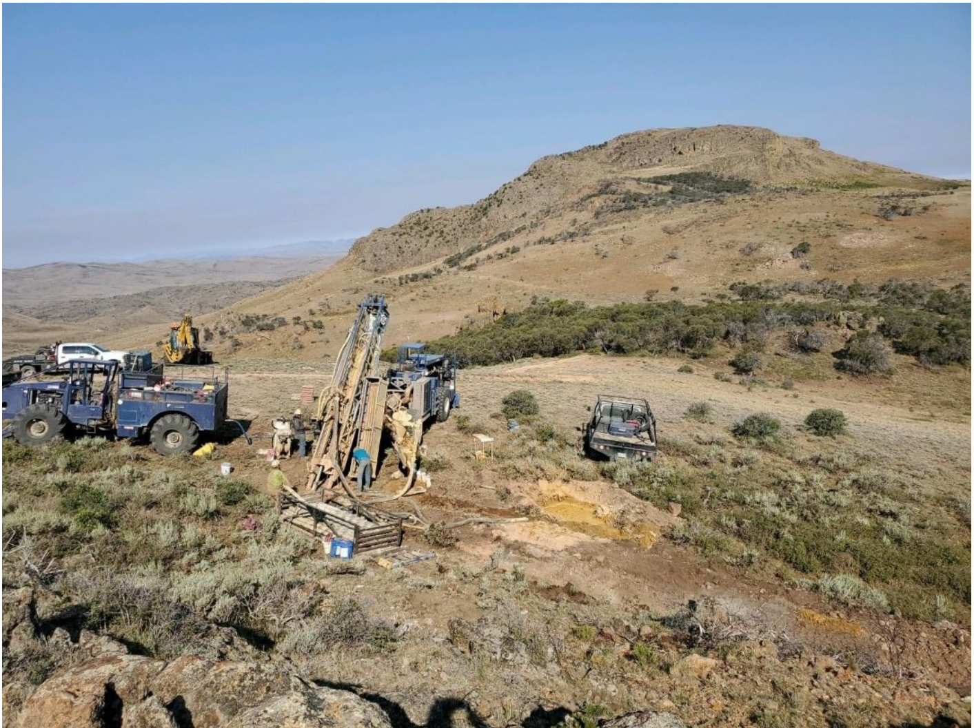
Figure 1 - Ongoing drilling at the White Rock Property, located in the southern part of the central mineralized area which extends under White Rock Mountain approximately 1.2 kms to the northwest of the drill rig. The first drill holes were against the mountain more than a kilometer to the north.
